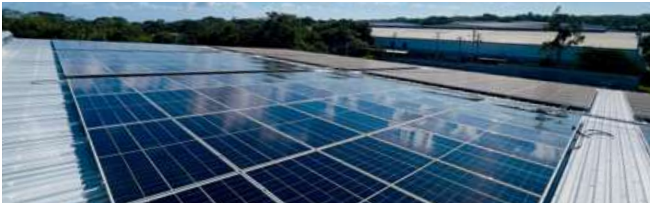
Solar Panels at HANSAE INTERNATIONAL, S.A.
